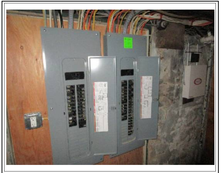
Basement - Electric Panels
