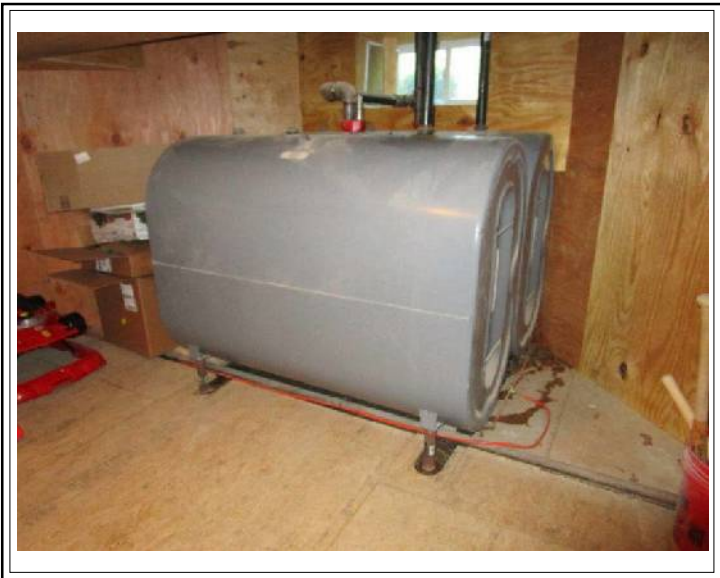
Basement - Oil Tanks
